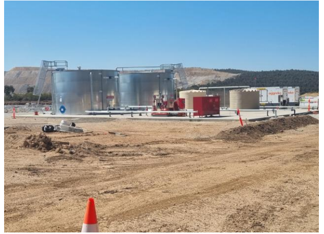
Photograph 7: Firefighting equipment as part of MOD9 facilities
