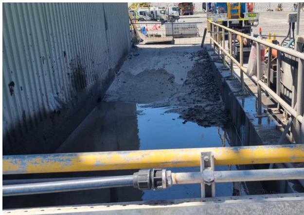
Photograph 14: Oil and grease separator
