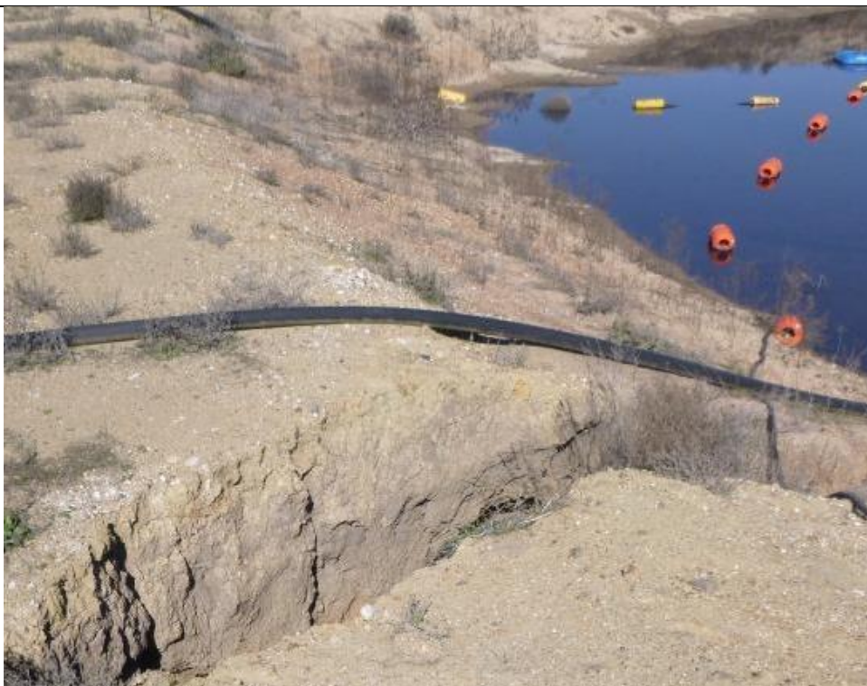
Photo 18 – Erosion of dam caused by incorrect location of pipeline running into the dam
