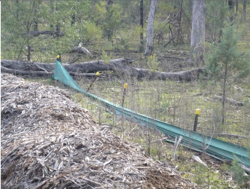
Photo 23 – Minor Sediment Fence maintenance required.
