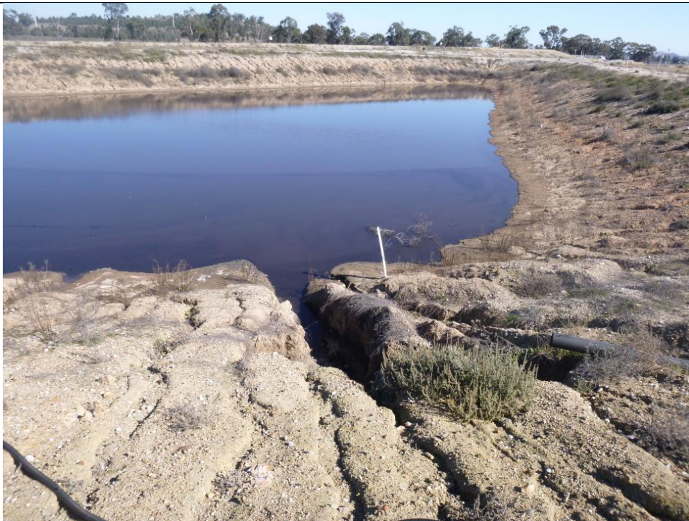
Photo 19 – Rilling and erosion of dam at TLO. Remediation work required.
