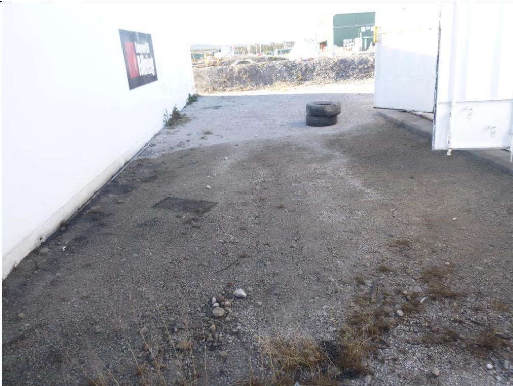
Photo 16 – Leakage in the fuel storage area. To be remediated.
