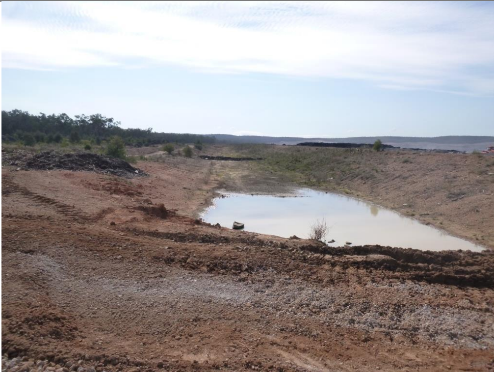
Photo 21 – A dam has been built towards the end of the clean water diversion drain. Additional water management work required in this area.
