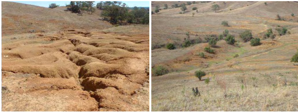
Photo E-8 Rill erosion in an ephemeral drainage line in the north and banks in the south of Sunshine
