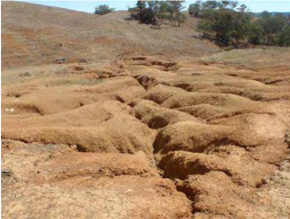
Photo 6.7 Rill erosion in an ephemeral drainage line in the north of the Sunshine BOA
