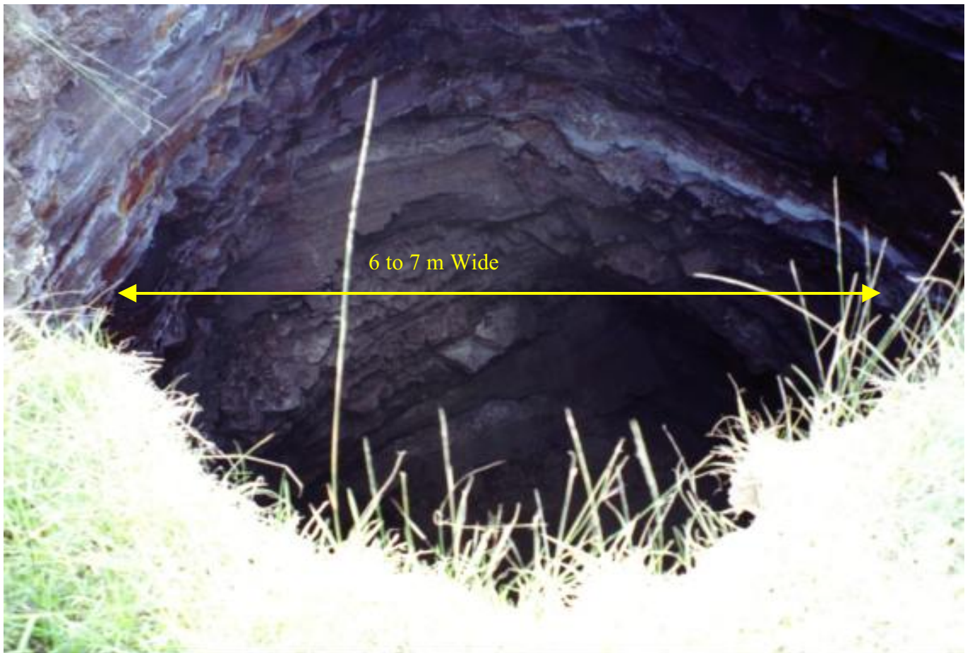
FIGURE 4.4. A pothole caused by collapse of the ground surface.
