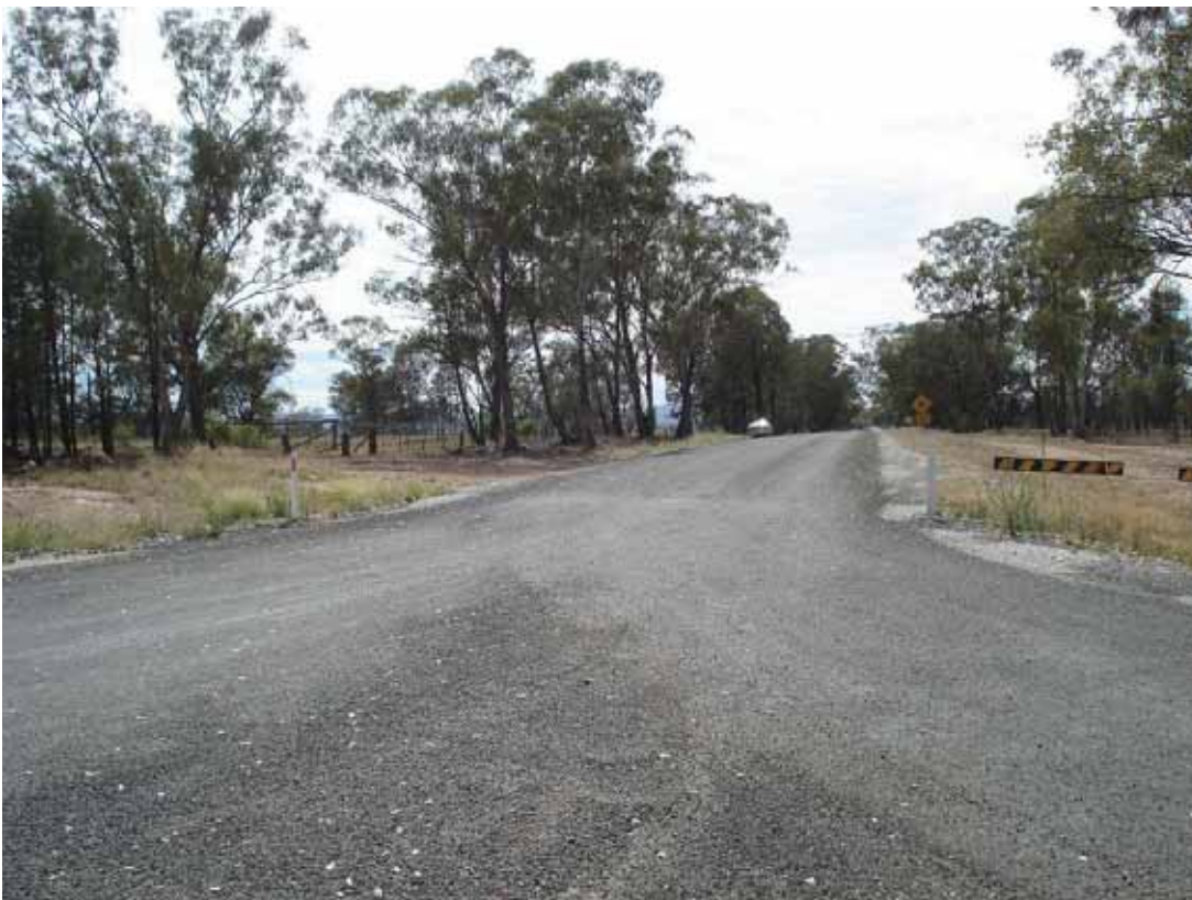
Photo 16 A pile of loose gravel collected in the centre of the intersection
