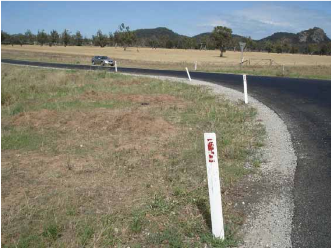
Photo 10 Damaged marker posts with reduced retro-reflectivity
