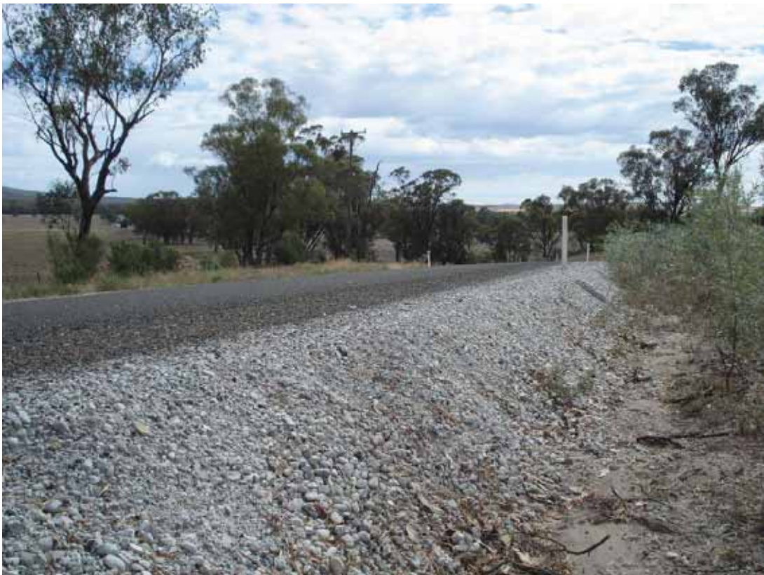
Photo 18 Batter slope steeper than the desirable 1:4 recommended
