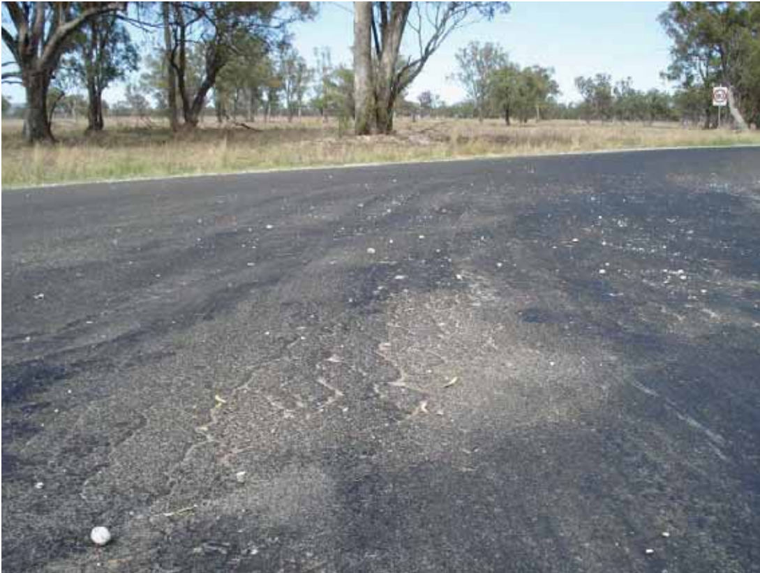
Photo 11 Fatigue cracking at the Manilla Road/Leard Forest Road intersection
