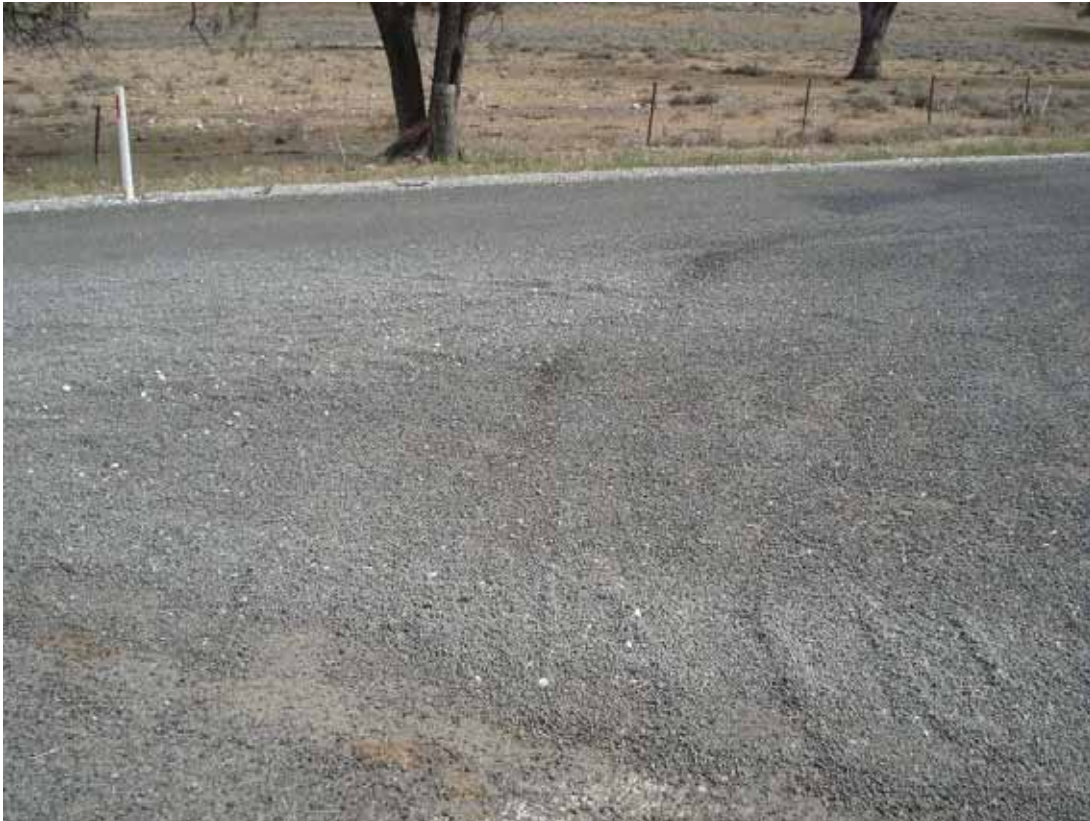
Photo 17 A pile of loose gravel collected in the centre of the intersection
