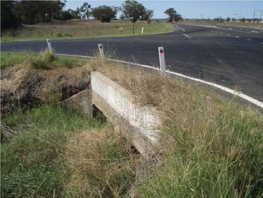
Photo 3 Poor maintenance of the drainage facilities
