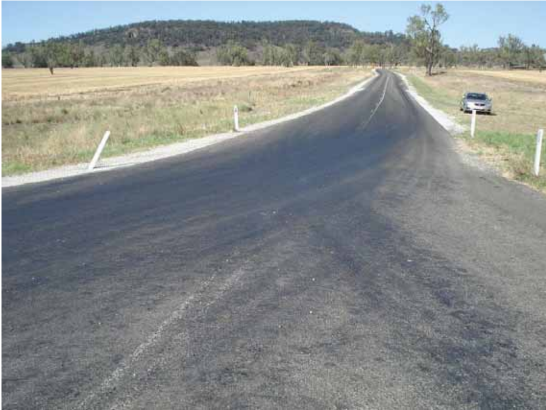
Photo 9 Faded centre line marking at the Manilla Road/Therribri Road intersection
