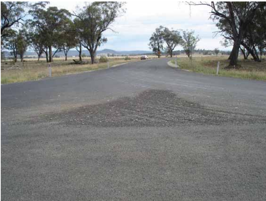
Photo 14 A pile of loose gravel collected in the centre of the intersection
