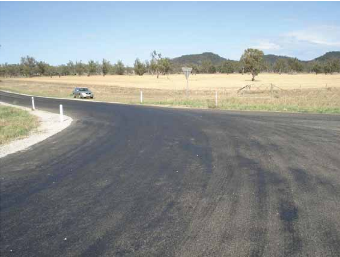
Photo 7 Bleeding at the Manilla Road/Therribri Road intersection
