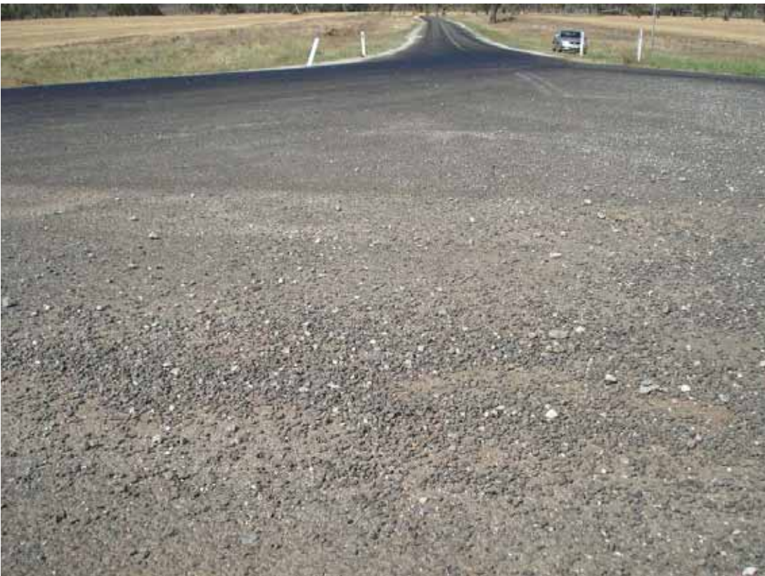
Photo 8 A pile of loose gravel collected in the centre of the intersection
