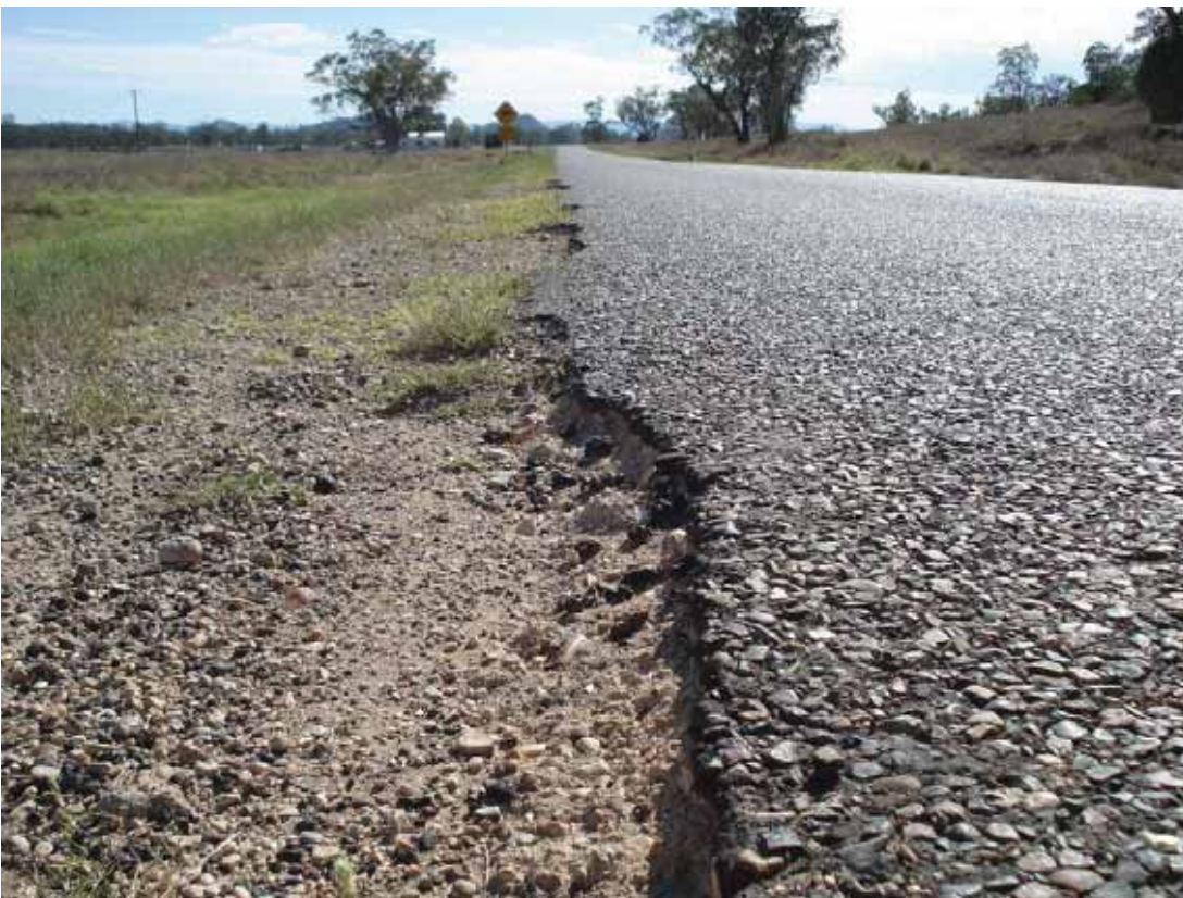
Photo 4 The edge drop-off, northern side of Manilla Road
