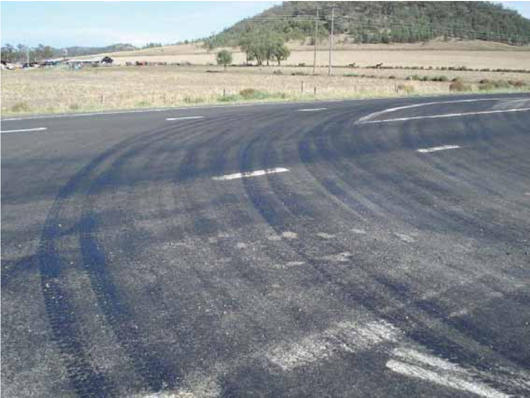
Photo 1 Bleeding at the Kamilaroi Highway/Manilla Road intersection
