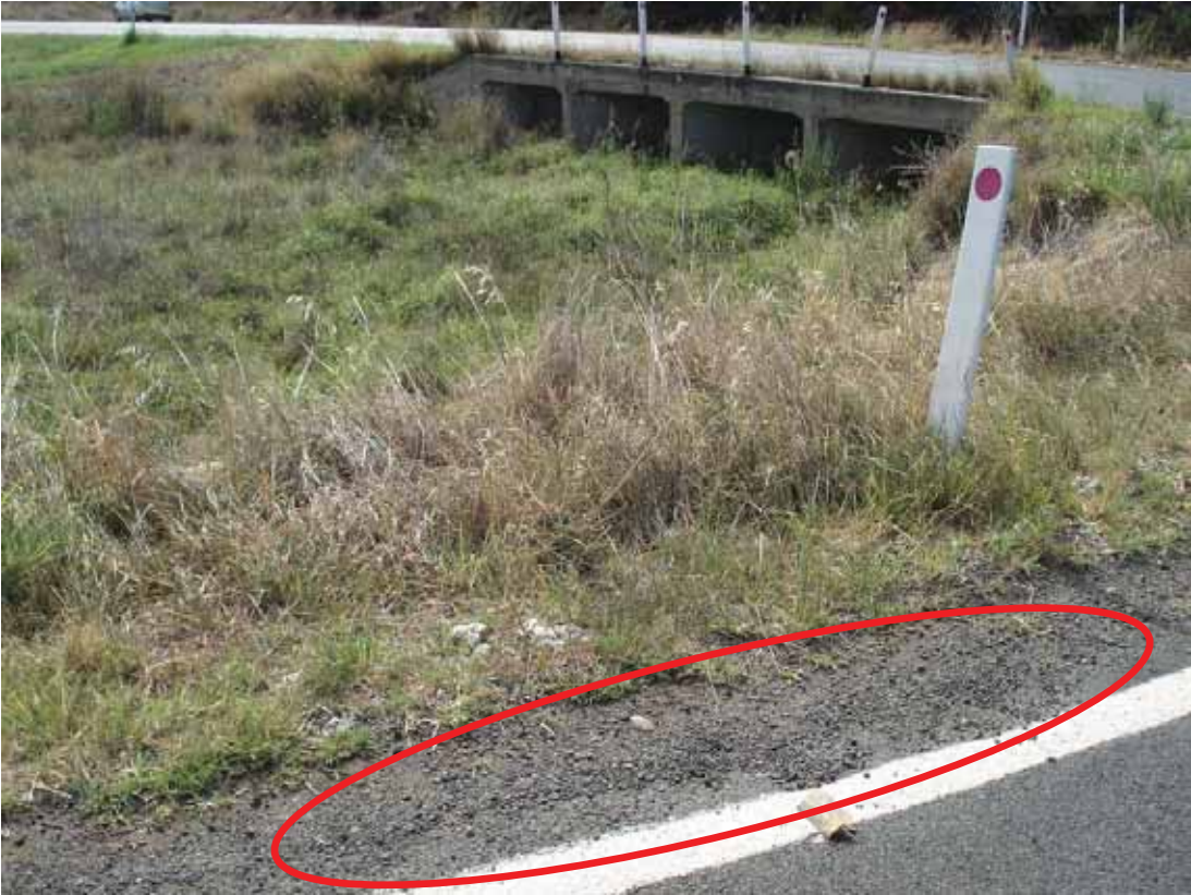
Photo 2 Loose gravel on the edge of the left turn auxiliary lane
