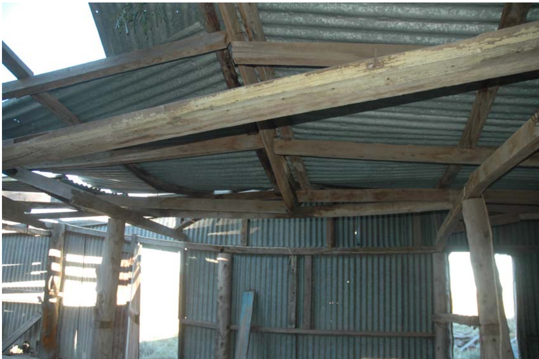
Figure 11 –Nagero 3 – Interior showing degradation of timber
